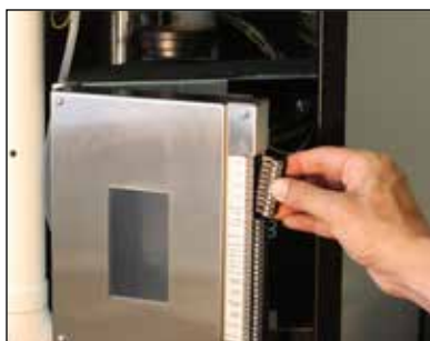
Line voltage load pump terminals
