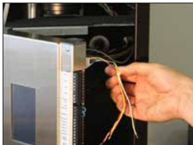
Line voltage leads for power supply, primary pump and VS output
