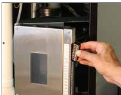
Line voltage load pump terminals
