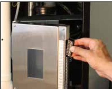
Line voltage load pump terminals
