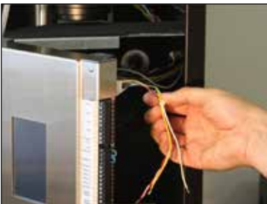
Line voltage leads for power supply, primary pump and VS output
