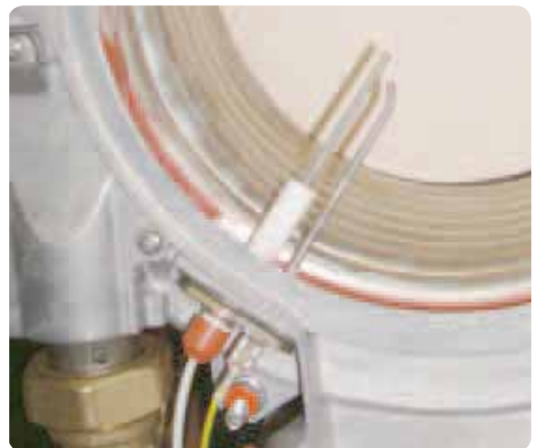
Figure 106 Inspecting ignition electrode
