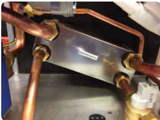
Figure 121 Removal of flat plate heat exchanger by loosening the four fittings
