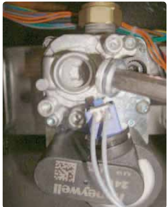
Figure 85 T-40 cap removed for adjustment
