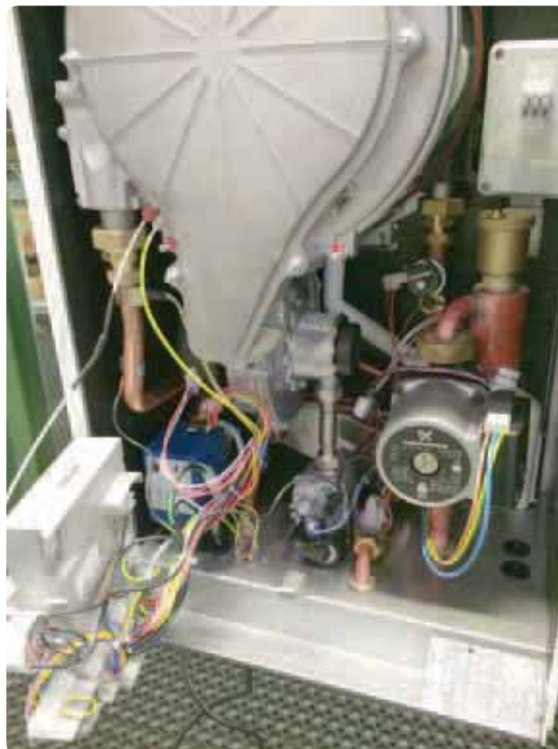
Figure 109 Boiler front panel removed
