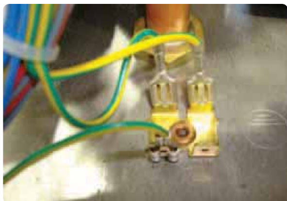
Figure 108 Ignition electrode grounding
