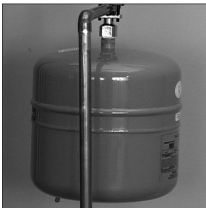
Figure 18 - The Thermal Expansion Tank should be pressurized with air to match the home's incoming water pressure.
